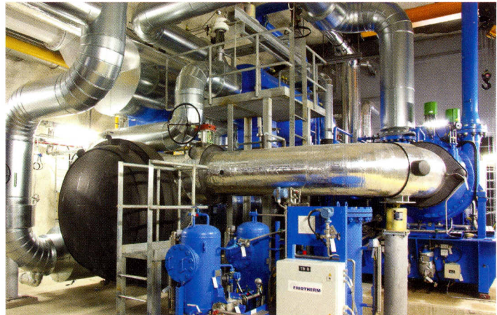
Katri Vala heat pump plant 2. Photo: Helsinki Energy
